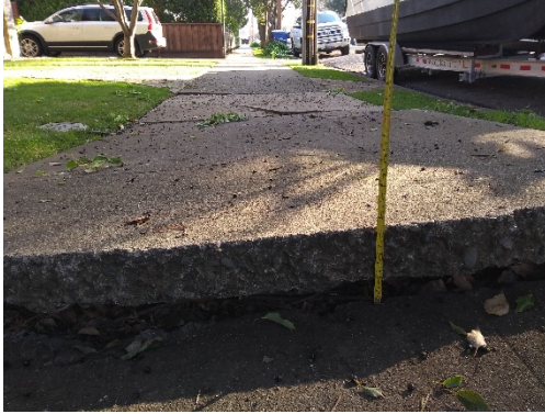
Fig. 3. 2019/2020 Grand Jury. Displaced sidewalk not on the sidewalk service list. 2020.
