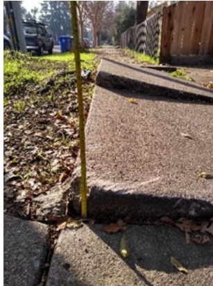
Fig. 7. 2019/2020 Grand Jury. Series of sidewalk segments displaced by more than four vertical inches. This segment of sidewalk has been on the “Sidewalk Service List” since at least March 2015.
